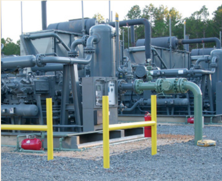
There are approximately 570 natural gas processing facilities in the United States, with more being built to support the increase in production from areas such as Pennsylvania.
